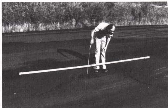
Figure 10.2. Thawing of ice-rich permafrost and the resulting thermokarst caused this road to settle which required repeated patching to keep the road in service.
