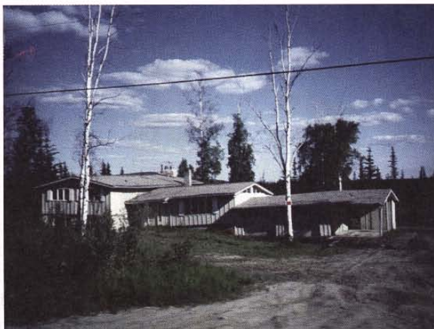
Figure 10.1. This house damaged by thermokarst in the Fairbanks area had to be abandoned.
