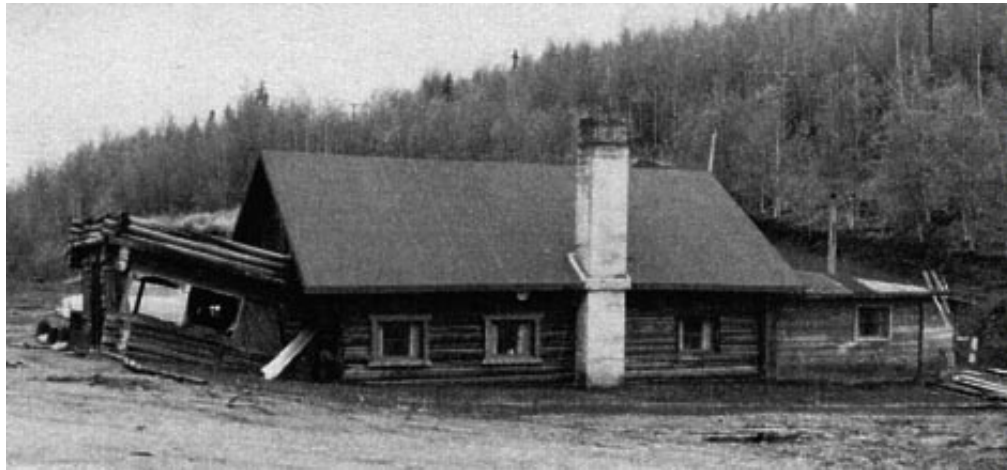
Figure 4. A permafrost-wracked house. 9
